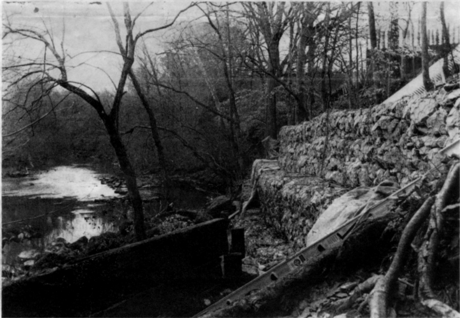
Figure 1. View south along river with gabion wall partially completed. Stockade wall at top right.
