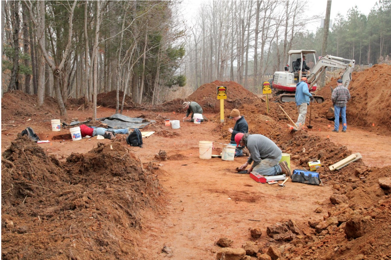
Figure 3.17. Excavating features and stripping topsoil along the high-pressure gas pipeline corridor. View to east.
